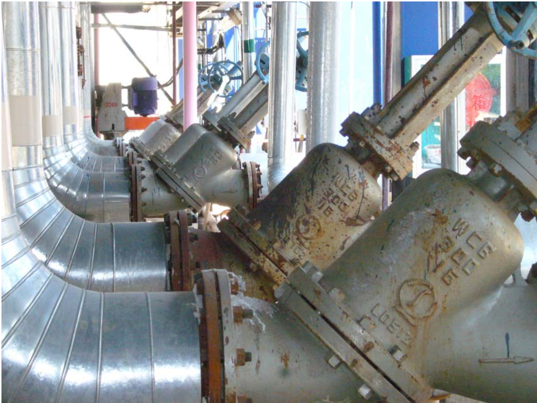
Alumina plant evaporation system
