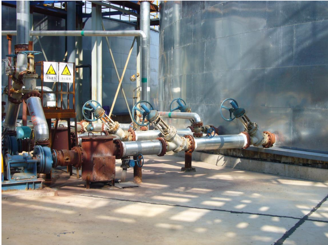
Thickener system in alumina plant
