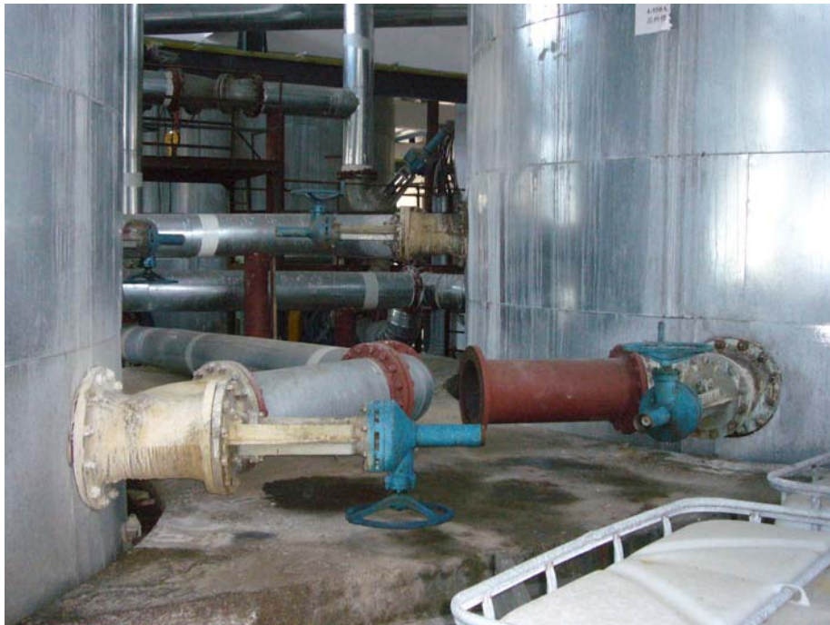
Pneumatic dumping valve used in alumina seed precipitation tank wall
