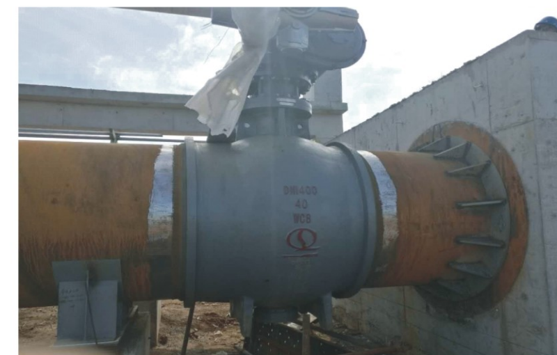
热力管网 Heat Supply Pipe Network
