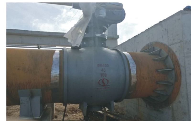
热力管网 Heat Supply Pipe Network
